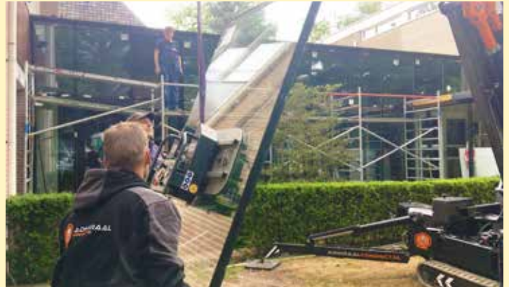
Installing the glass facades in the part of the TUA that is being renovated. This made the building glass-tight.
